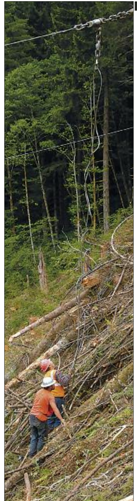
STRAIGHTENING OUT THE LINES is Eric Wisti working with Jayson Reynoso in the brush on the Wisti Logging downhill yarding side.
